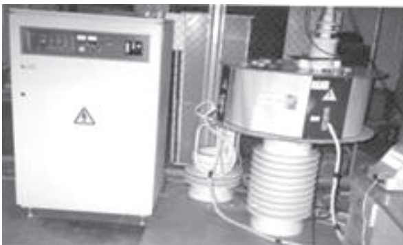
Fig. 9. Frequency converter and resonance circuit of transmitting high-voltage transformer with electrical power of 20 kW, 10 kV.
